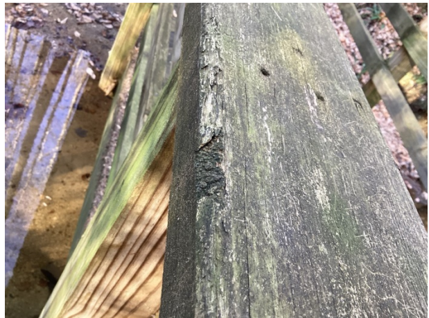
Longer bridge wood deterioration
