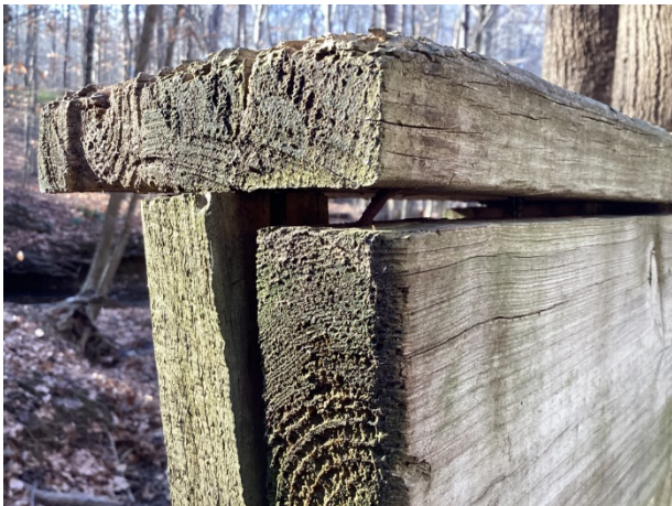
Shorter bridge rusted and loose connection
