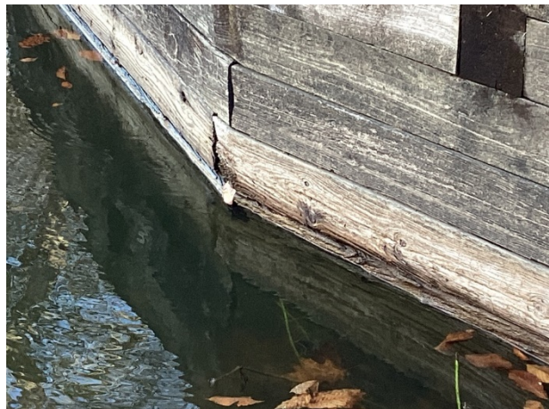
Wall wood rot
