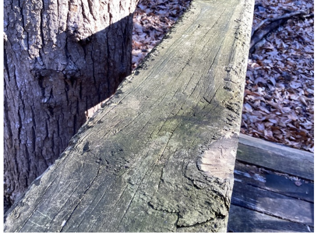
Shorter bridge wood deterioration
