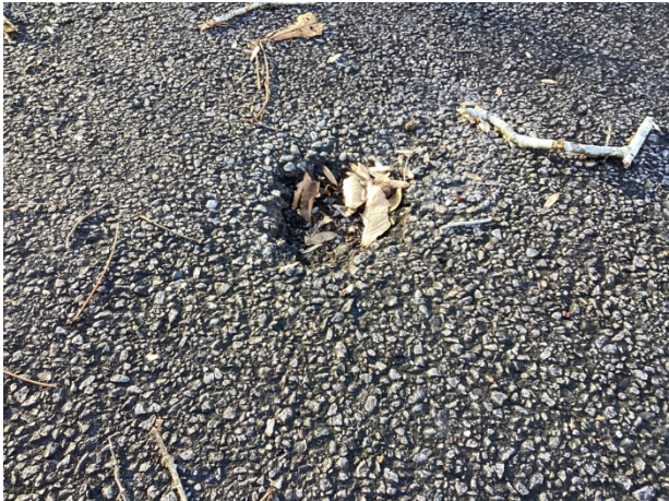
Pavement pothole formation
