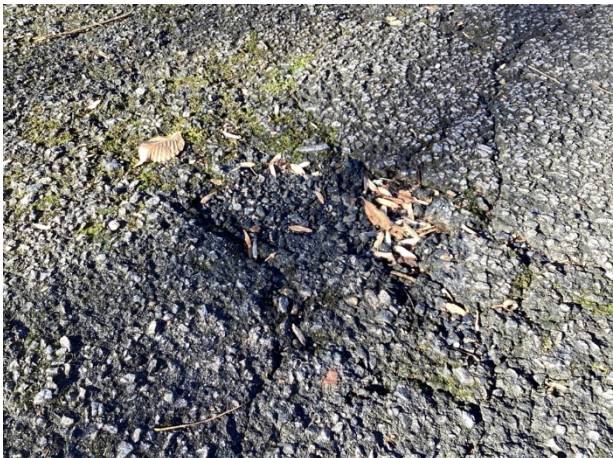
Pavement pothole formation
