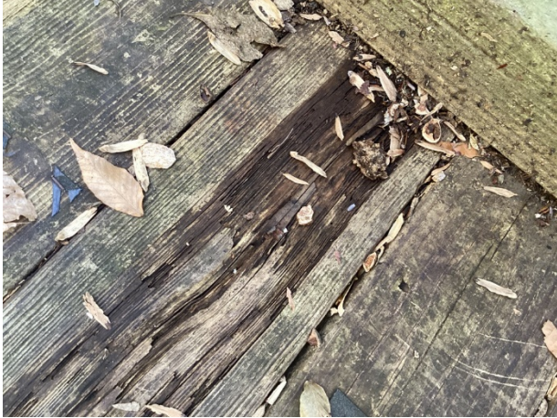
Shorter bridge wood rot
