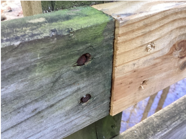
Longer bridge rust
