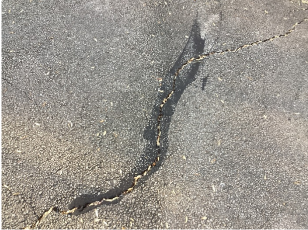
Pavement cracks with repairs
