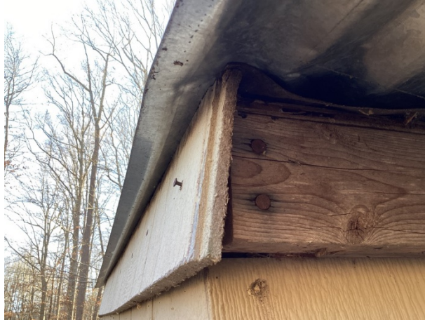
Rusted and loose fastener
