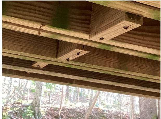
Longer bridge rusted fasteners
