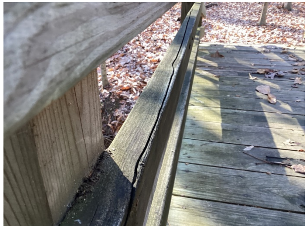
Longer bridge wood splits
