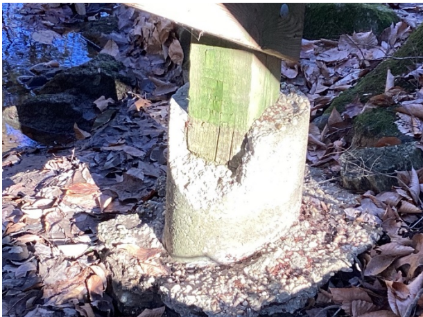
Longer bridge concrete footing deterioration
